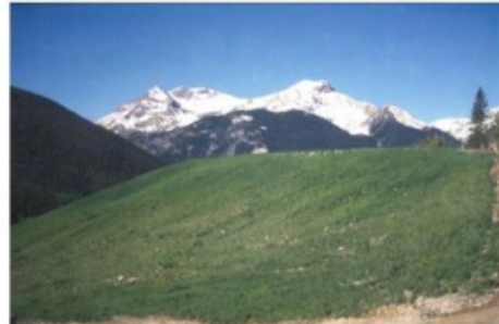
Mayflower Tailings pond 1, 1995 (after) – SGC moved the impoundment toe back from Boulder Creek and the highway to minimize the potential for erosion and migration. SGC flattened the side slopes to increase stability and potential for re-vegetation, regraded to promote drainage, capped with subsoil, and seeded.
