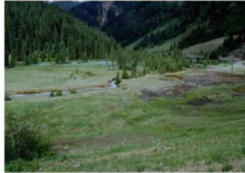
Lead Carbonate Tailings, 1994 (after) – SGC relocated 27,000 cubic yards of tailings to Mayflower Impoundment #4, regraded, neutralized, and reseeded the area.
