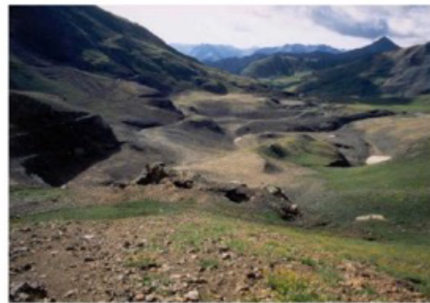
Sunnyside Basin, 1996 (after) – SGC placed 240,000 cubic yards of clean fill to cover the Lake Emma subsidence area and to create positive drainage, contoured the area, and seeded.
